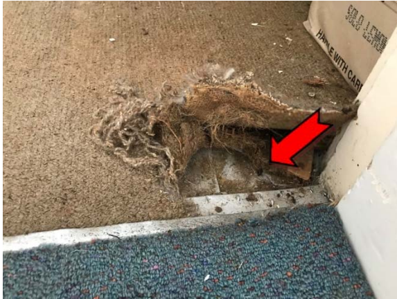
Photo 7. Interior, occupational therapy room, beneath carpet, throughout – asbestos-containing vinyl floor tiles.
