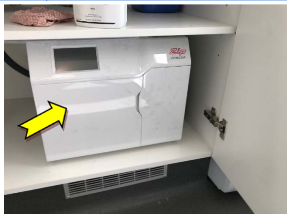
Photo 18. Interior, kitchen, under sink, hot water heater – suspected SMF internal insulation material.
