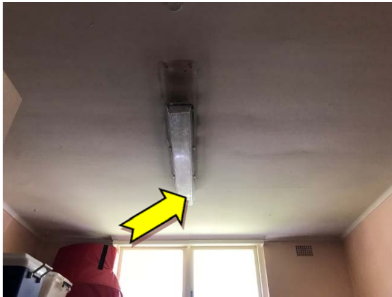
Photo 21. Interior, throughout, double tubed fluorescent light fitting – suspected PCB-containing capacitors.
