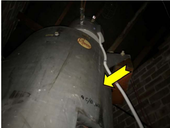
Photo 19. Interior, kitchen, ceiling space, hot water heater – suspected SMF internal insulation material.
