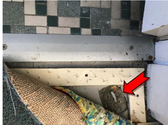
Photo 8. Interior, foyer, beneath carpet, throughout – asbestos-containing vinyl floor tiles.
