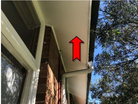
Photo 1. Exterior, throughout, eaves – asbestos-containing fibre cement sheeting.
