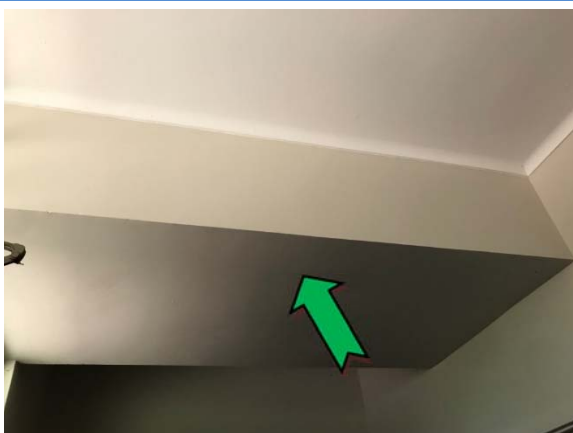
Photo 11. Interior, female toilets, high level boxing – non asbestos-containing fibre cement sheeting.
