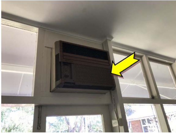
Photo 25. Interior, western elevation, air conditioning unit, unknown refrigerant – suspected ozone depleting substances.
