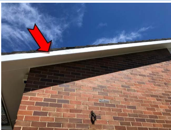
Photo 5. Exterior, throughout, gable verge lining – assumed asbestos-containing fibre cement sheeting.
