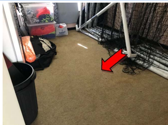
Photo 12. Interior, room 3, beneath carpet, throughout – asbestos-containing vinyl floor tiles.
