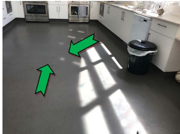
Photo 16. Interior, kitchen, floor – suspected non asbestos-containing sheet vinyl; non asbestos-containing vinyl floor tiles and screed (beneath sheet vinyl).
