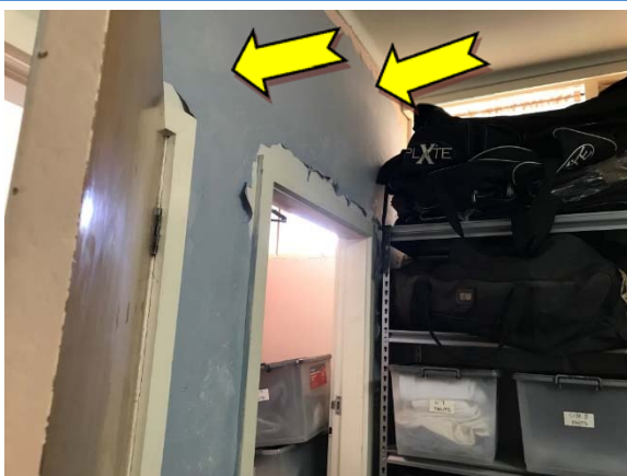
Photo 23. Interior, occupational therapy room, walls – suspected lead-containing blue upper and orange lower coloured paint systems.
