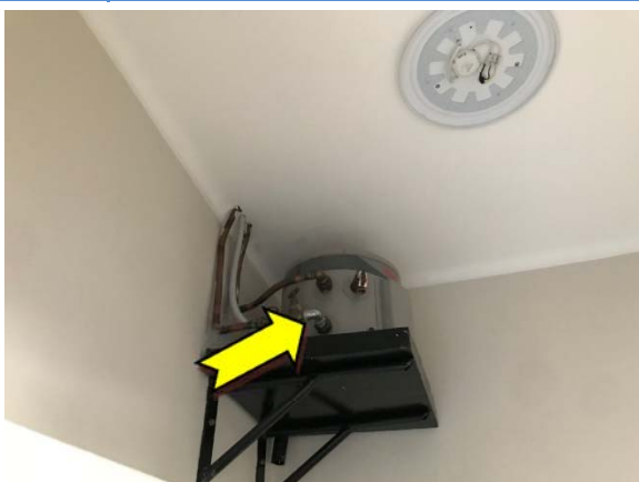
Photo 17. Interior, female toilets, hot water heater – suspected SMF internal insulation material.
