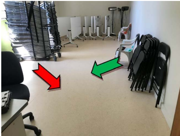
Photo 15. Interior, room 1, floor, throughout – non asbestos-containing sheet vinyl and asbestos-containing vinyl floor tiles (beneath sheet vinyl).
