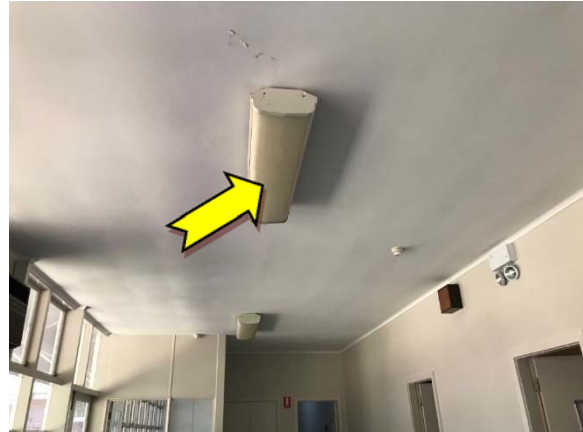
Photo 20. Interior, throughout, quadruple tubed fluorescent light fitting – suspected PCB-containing capacitors.
