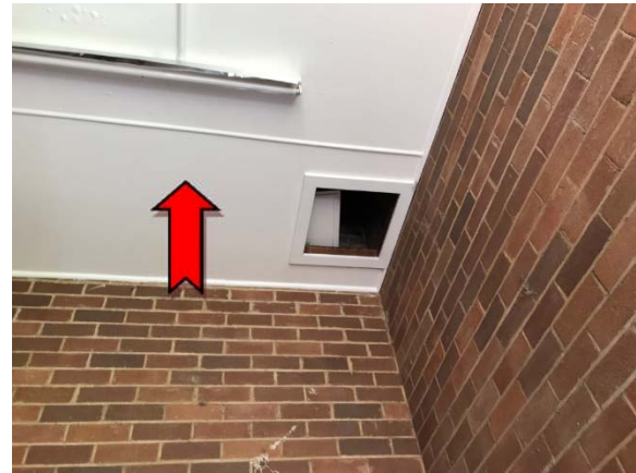
Photo 4. Exterior, north elevation, awning – assumed asbestos-containing fibre cement sheeting.
