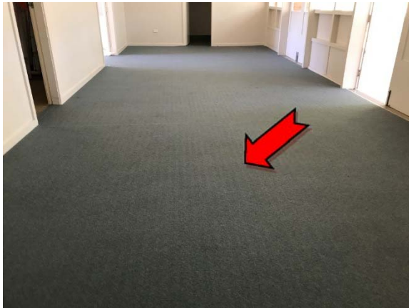
Photo 9. Interior, open room, beneath carpet, throughout – asbestos-containing vinyl floor tiles.
